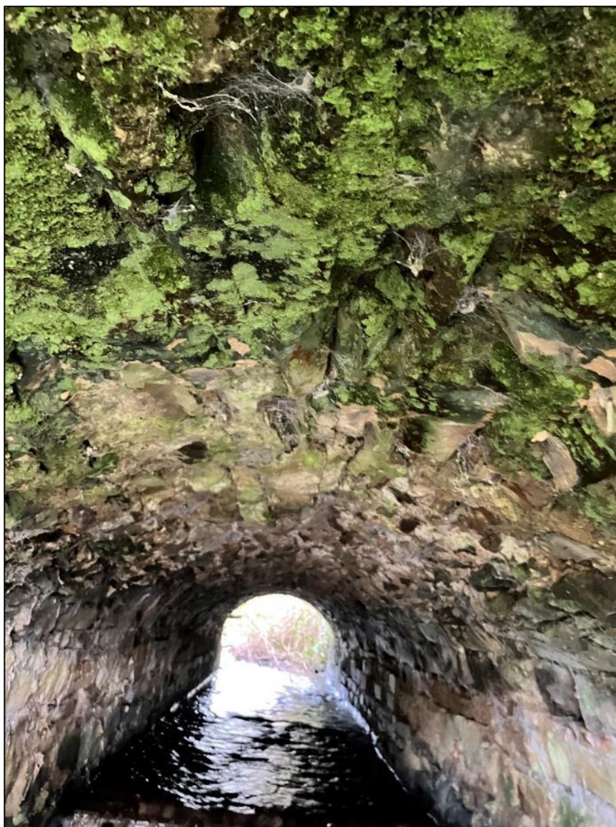
Image 13: Barrel under bridge.
