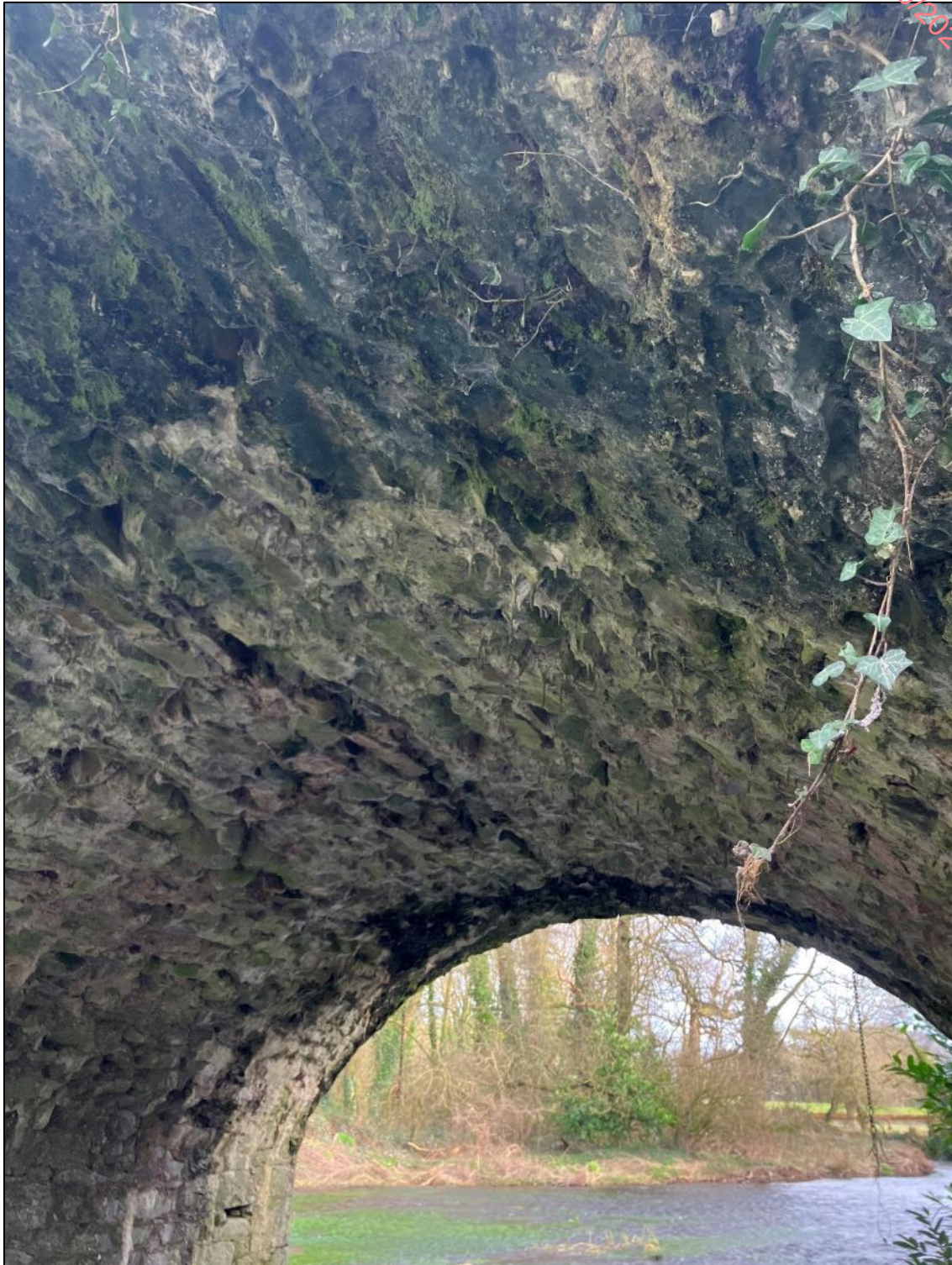
Image 4: Cavities at apex of barrel of Arch 1.
