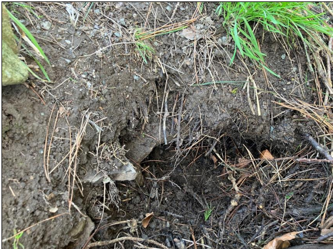
Image 15: Precast concrete drainage pipe.
