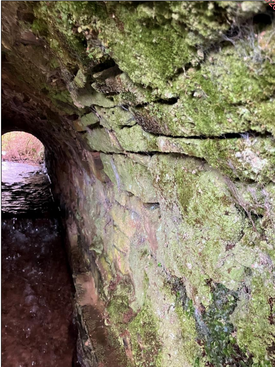
Image14: Some joints in masonry require filling.
